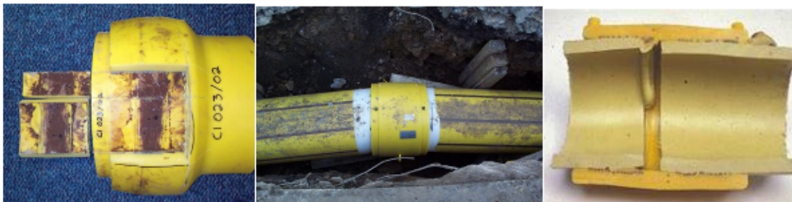
Figure 8: Examples of electrofusion coupler joint failure: gross contamination (left), gross misalignment (centre), and section through misaligned joint showing constrained leakage path (right)
