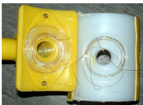
Figure 9: Electrofusion saddle joint failure causing complete separation of top tee from pipe
