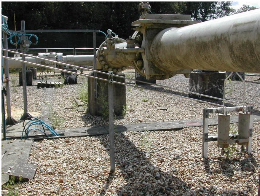
Figure 4.8 – Transmitter Impulse Lines and Catchpots
