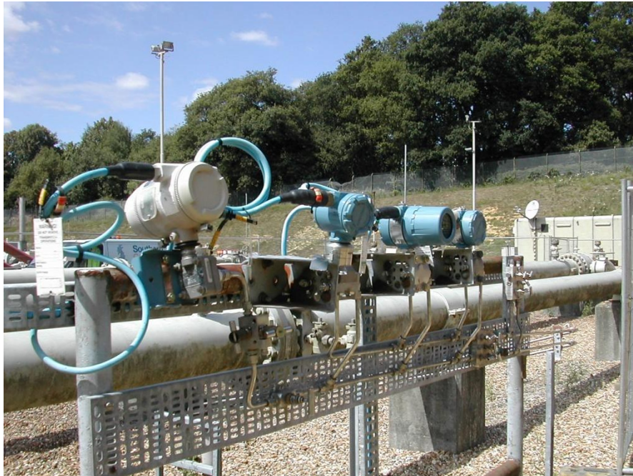
Figure 4.7 – Transmitter Mounting Rack
