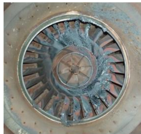
Figure 11: Flashback damage to burners has been linked to high levels of higher hydrocarbons.
